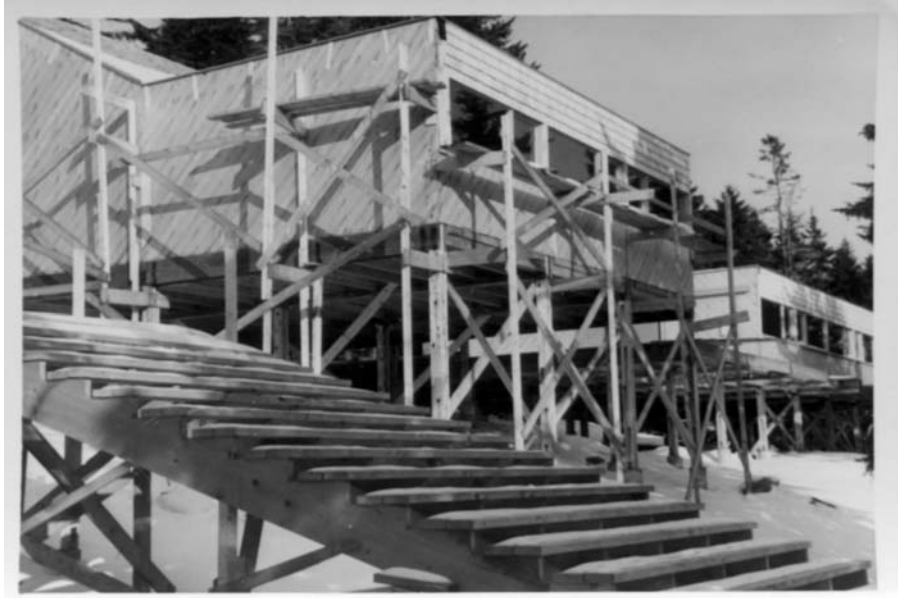
Main stairs and metals studio under construction, 1960–61, from Discovery: Fifty Years of Craft Experience at Haystack Mountain School of Crafts from the University of Maine Press.
