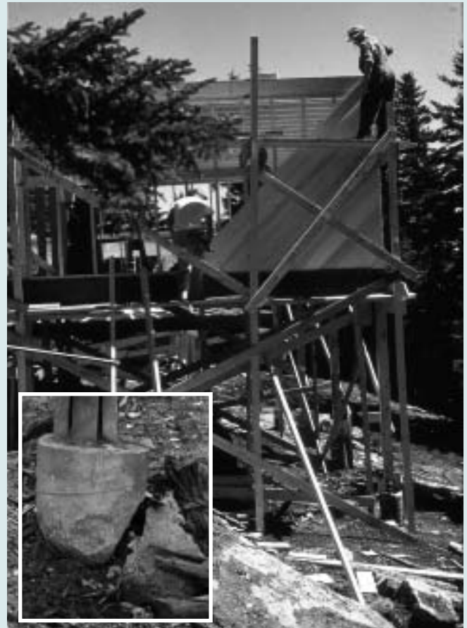
These images show early campus construction c1960 and some of the damage (inset) to be addressed with the grant from Save America's Treasures. Vital restoration projects at Haystack will be supported by this award, in addition to replacement of supporting posts and piers, projects will include the replacement of rotted carrying timbers and repairing damage to roofs and windows.
